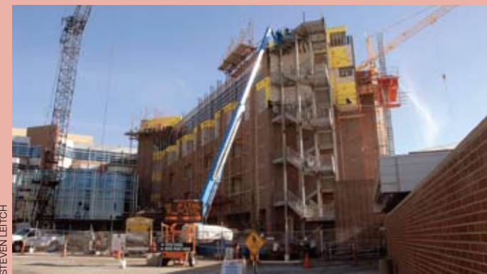
THE PRESENT An average of 250 construction workers per day have logged 390,000 hours on the project. Another 200,000 man-hours are expected before the job is complete. They are currently installing the electrical, plumbing and other support systems. By July 2009, all of the finishing touches will be complete.
