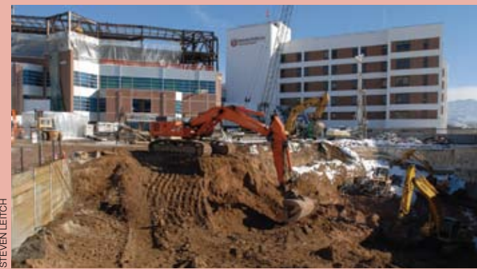
THE PAST 90,000 cubic yards of soil were removed to create the lower levels and foundation of what is to be the new West Pavilion of University Hospital. Digging began in July 2006 and exactly two years later the last piece of structural steel was added to the building that quickly occupied the hole in the ground.
